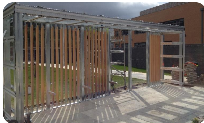
Above: One of the shelters during installation before the Trespa cladding was fitted
